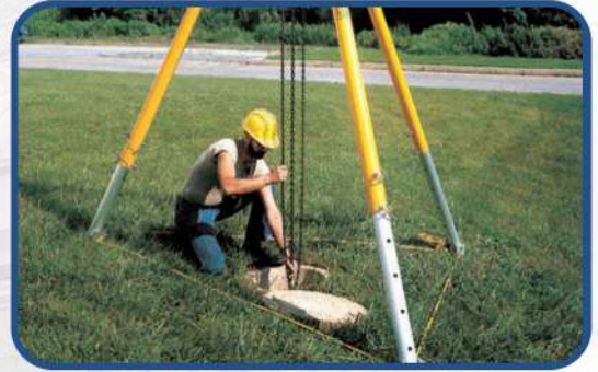
A worker using a Verkrönn Tripod with Mud Feet to lift a manhole cover single handedly.
